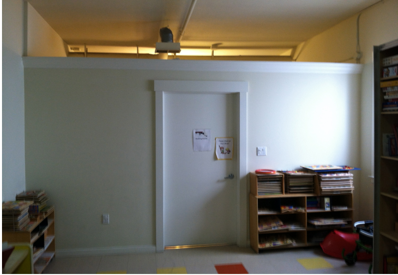
Figure 39. Doorway leading from main hallway to waiting room. Also shows gap in wall
