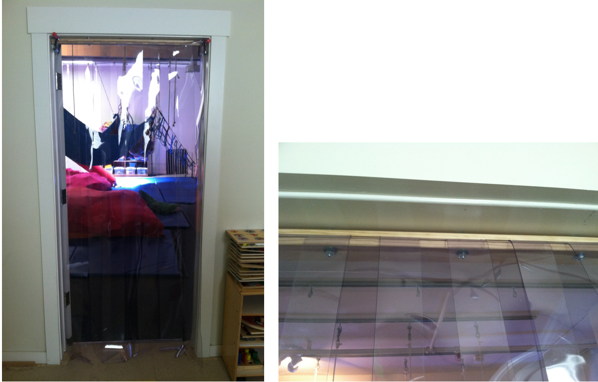
Figure 28. (left) The working model of the PVC flap door temporarily installed in the doorway to the front gym. (right) The method of attachment still allows for the existing door to be shut.
