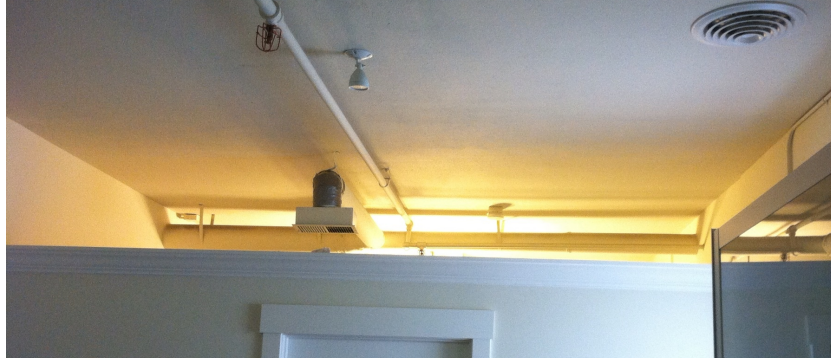
Figure 7. The gap in the wall dividing the main hallway and the waiting room, taken from the main hallway. Note that the air duct and vent are completely on the waiting room side and the red sprinkler is on the hallway side. http://www.acousticalsurfaces.com/noise_barrier/vinylbar.htm?d=14
