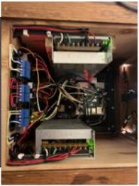
Interior of Completed Electronics Bay
