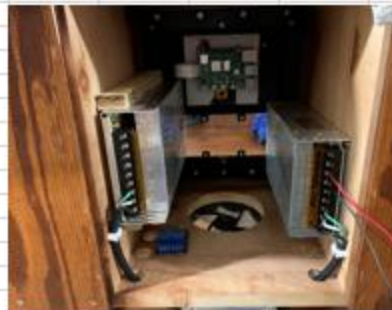
Power Supply Units Mounted
