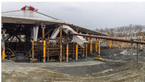
VERTICAL STRUCTURE: CONCRETE V-SHAPED PIERS AND FOUR LARGE ABUTMENTS TRANSFER LOADS TO GROUND
